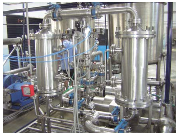
A view of the Membrane Processing Unit at Integrated fruit juice processing plant, Litan, Imphal - the plant was setup by CFTRI for MATA Foundation
